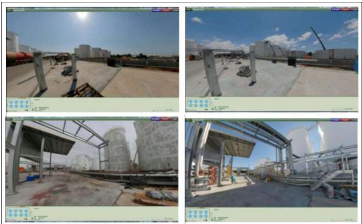
Figure 2-20 The VR application showing the sequence of construction at Pacific Terminals Australia (PTA), starting from the top left image to the bottom right image (Maynard et al., 2011).
