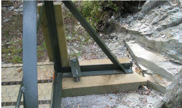
Figure 4.1g-8: is a close-up of the far end of the bridge in Figure 4.1g-7. One can see where the substantial rock on which the bridge rests has had to be sawn back to eventually accommodate the bridge structure.
