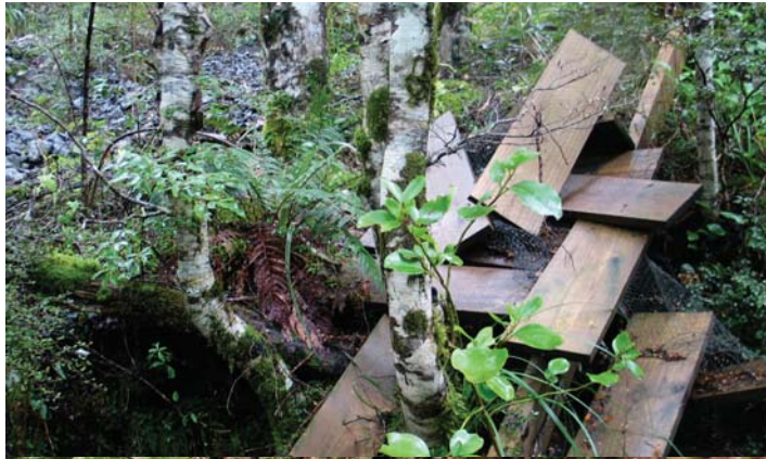
Figure 4.1g-5: shows a small bridge that has been swept downstream in a flood and discarded for some time. It should also be noted that because this structure is registered in the VAMS database its destruction would have been noted during routine inventory checks.
