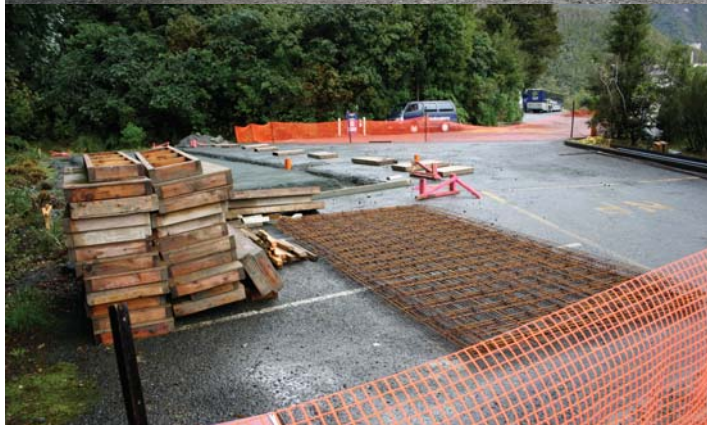
Figure 4.1c-10: Construction site directly beside the passenger terminal and is part of ongoing building projects.
