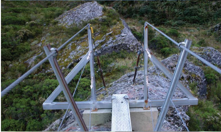
Figure 4.1g-3: shows a rough concrete footing poured to form an even surface on which to fix a standard bridge solution across the upper West Matukituki River.
