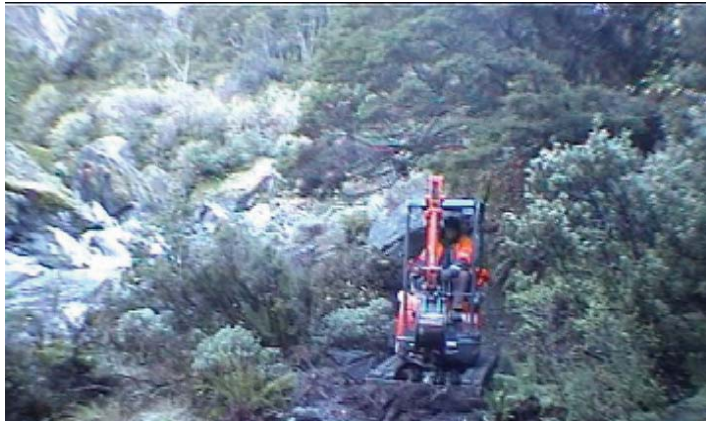
Figure 4.1g-9: is a still from video footage taken of a digger working on the upper Rob Roy Glacier track. Difficulty of access meant the digger was helicoptered in.
