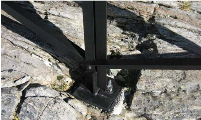
Figure 4.1g-1: shows one of the many footings cut out of the rock so the recently replaced French Ridge Hut can be bolted to the ground. In the lower front of the image you can see the saw marks that cut into the rock.
