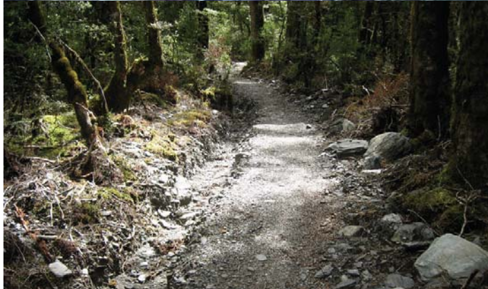
Figure 4.1g-10: is an example of a track made by digger. Its width and form, while intended for people to walk on, is that of a vehicle track set by the obvious requirement that a digger must be able to travel along it during its construction.
