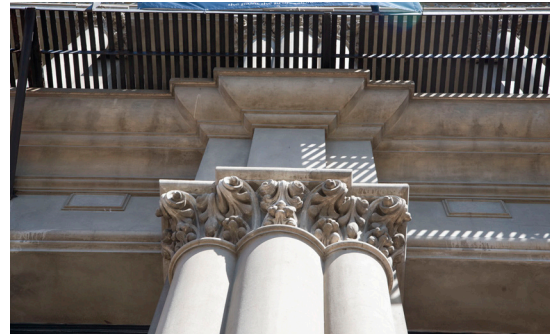
Figure 36 Decorative cornices found on one of the historical buildings in the Warehouse Precinct (image by author).
