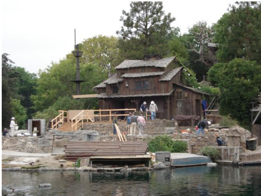
Figure 22. No effort is made to hide the construction taking place on Tom Sawyer Island (Source: Author).
