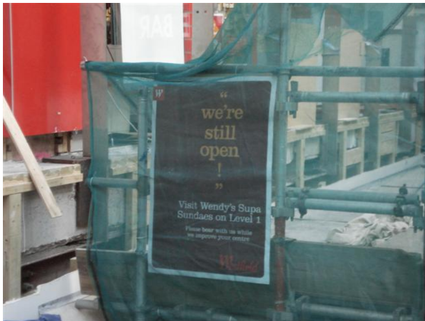
Figure 35. These renovations of a Wendy's Ice Cream store at St Lukes are a little harder to screen from the shoppers eye (Source: Author).
