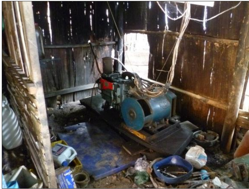
Figure 5.6 Generator that supplies around 30 Prek Svay families with electricity
