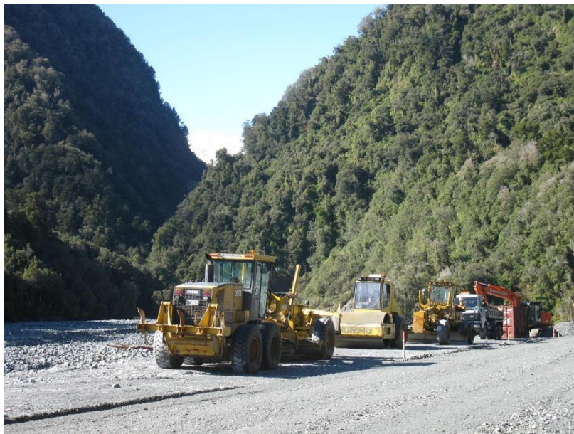
Photograph 15: Heavy machinery working on Franz Josef glacier access road (Photo Credit: Jude Wilson)
