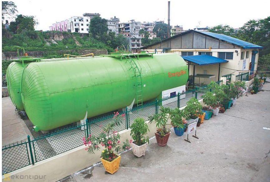
Figure 2-18: KMC's bio plant at Teku has started producing fuel.
