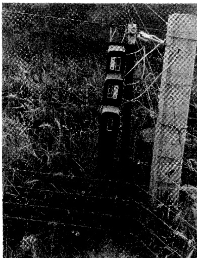
Use ordinary electric fuses at central points and find and disconnect short-circuited wires. Note the tin rain shields.
