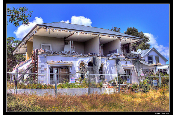
Figure 1: Godley House, post-earthquake (Geoff Trotter)
